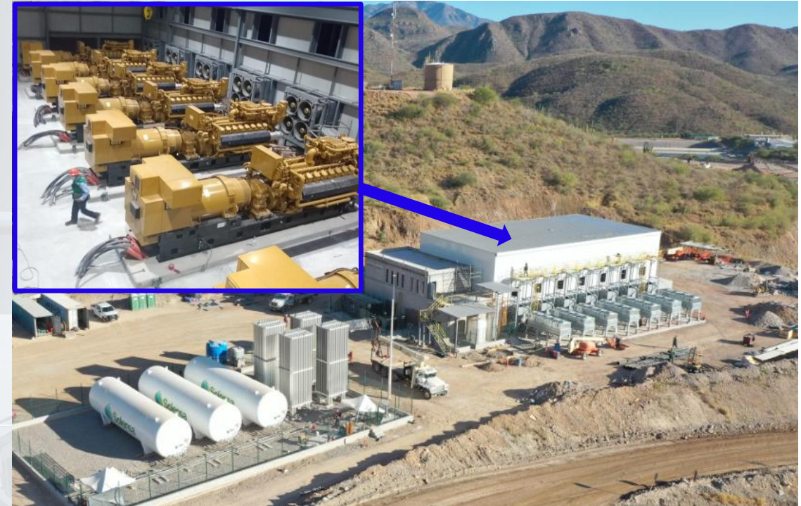
Santa Elena's new 12.4MW LNG Power Plant
